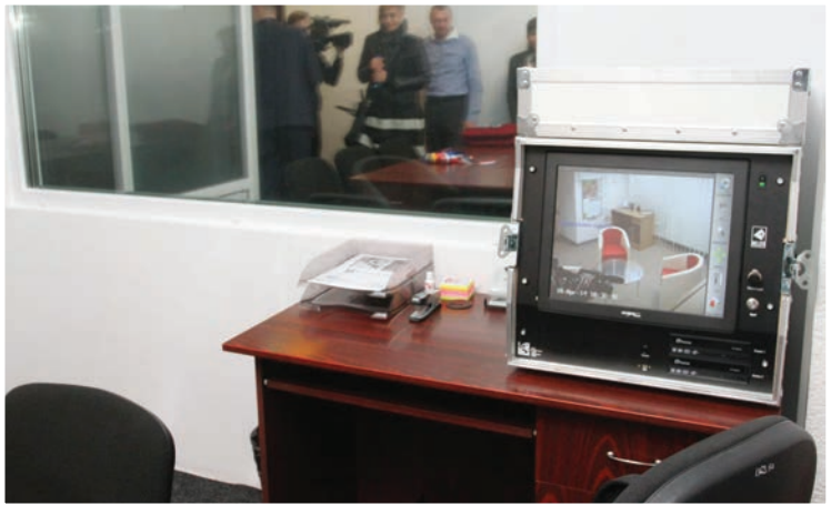
The „technical premise“ in the room in Cluj-Napoca, Cluj Department
